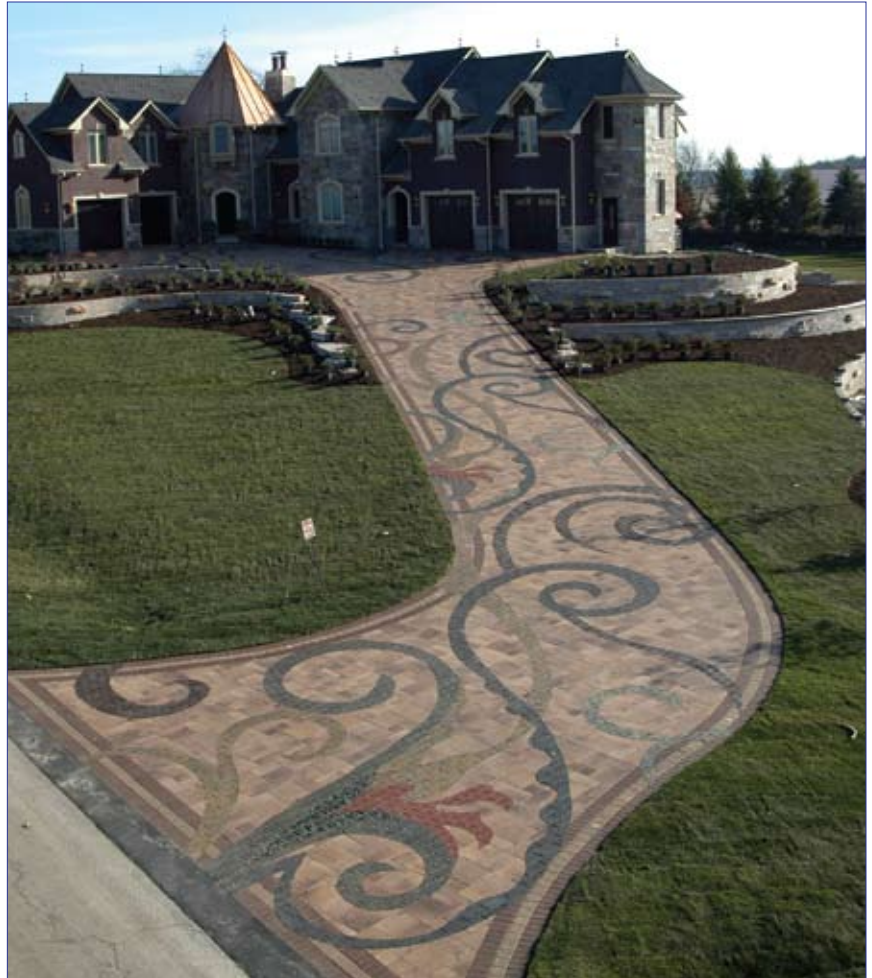
The 6,500 sf (650 m 2 ) driveway utilized eleven different colors and textures of concrete pavers to create this vine-like mural.
